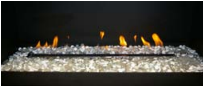
Figure 27a. Operating gas fireplace with firestones surrounding burner tray.
