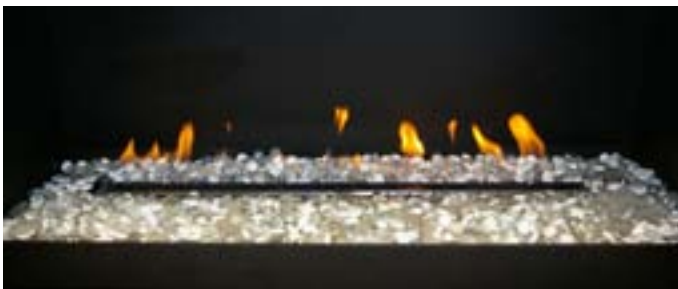
Figure 26a. Operating gas fireplace with firestones surrounding burner tray.
